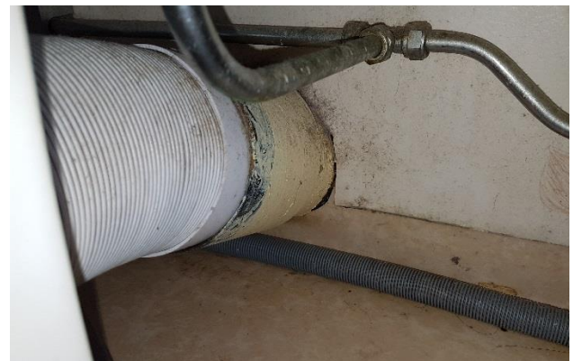
WC connection with no sealant.
