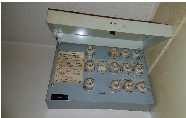
The distribution boxes have screw-in plug fuses
